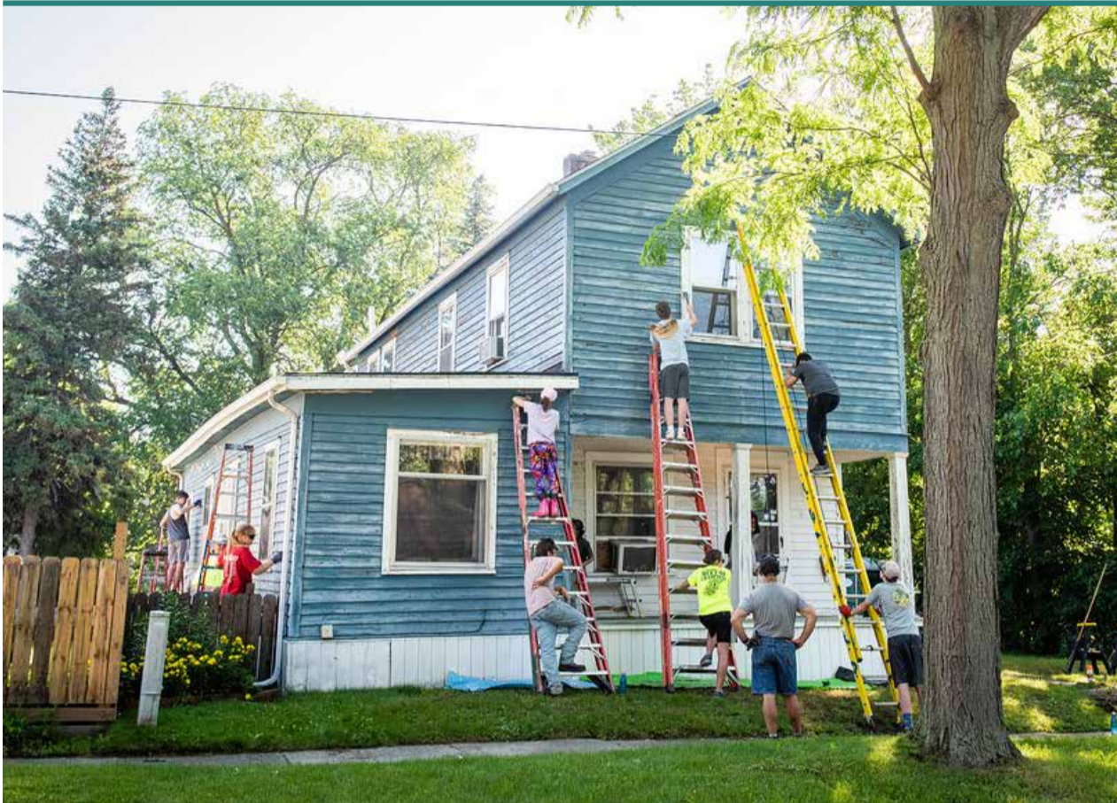
HIGH SCHOOL-AGED YOUTH PERFORM EXTERIOR REPAIRS AND PAINT A HOME IN SAGINAW DURING A WEEKLONG MISSION IMMERSION EXPERIENCE
